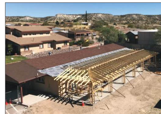
From laying the concrete for the foundation to building the structure's framework to installing the rafters, construction of the WTC Patio is going to provide a vital new outdoor space for activities.
